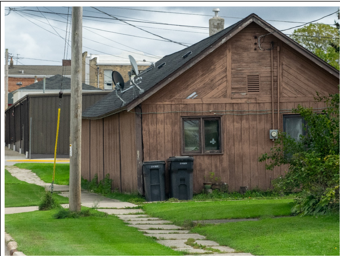
516 Steele St.- is showing deterioration, including sagging roof, deteriorating siding in need of paint, deteriorating public sidewalk;
